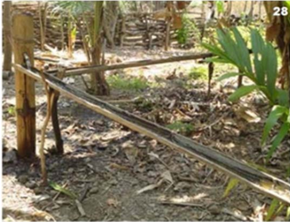
Picture left: Self-made bamboo type plumbing for water supply system within the village of Vativou, Liquiça District; low efficiency and pollution risks.
